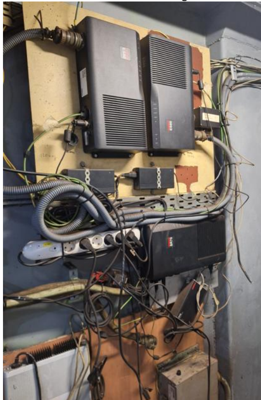
Distribution of system in sonar room
