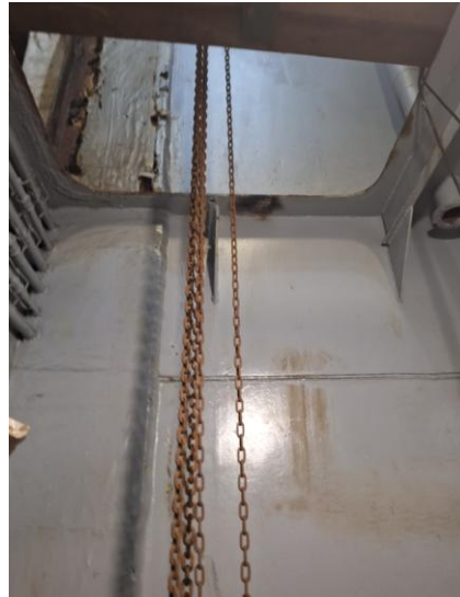
Works done on sonar room to install the hull unit (lower deck)
